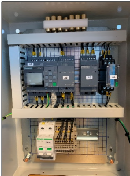
Plugs inside Insulation guard
