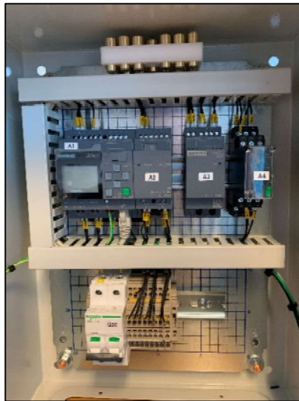
Plugs inside Insulation guard
