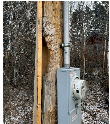
REC power pole damaged by a black bear
