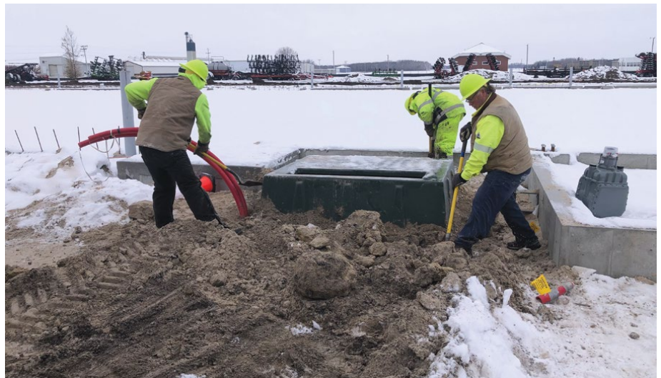
Linemen preparing a basement for a transformer to be set for a new service
