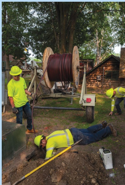
Teamwork comes into play when threading hundreds of feet of cable underground.
