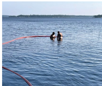
REC linemen diving to connect innerduct to the directional boring machine to be pulled back onto the island
