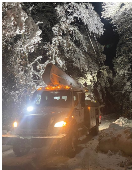
REC crew using a spotlight to locate snow covered power lines.
