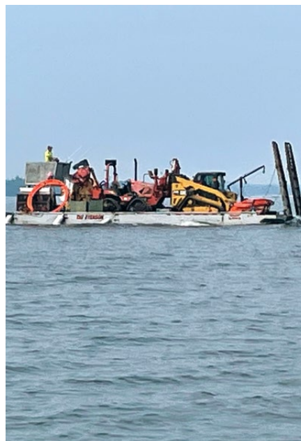
Crews transport equipment from the Mainland to Oak Island for a line change conversion.
