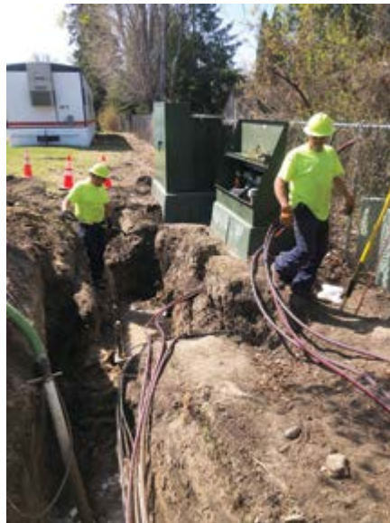
Ross Nelson and Chad Nelson working on a line change for the Roseau school expansion.
