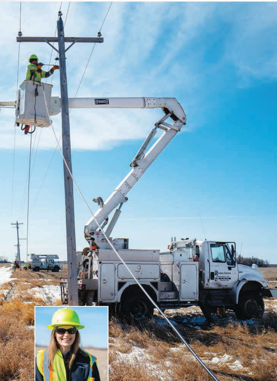
An REC lineworker drills a hole to prepare the placement of a fiber cable trunnion. Inset: Stacy Rose displays a trunnion used to hold the fiber line along the power poles.
