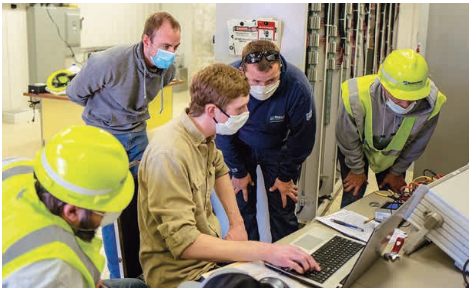
(Left to right) Joe Hensel, Patrick Rickenbacher, Nick Gellerman, Jared Thompson and Jason Bjerke work together to tune the new ripple injection system at the Wilton substation from the adjacent control house.
