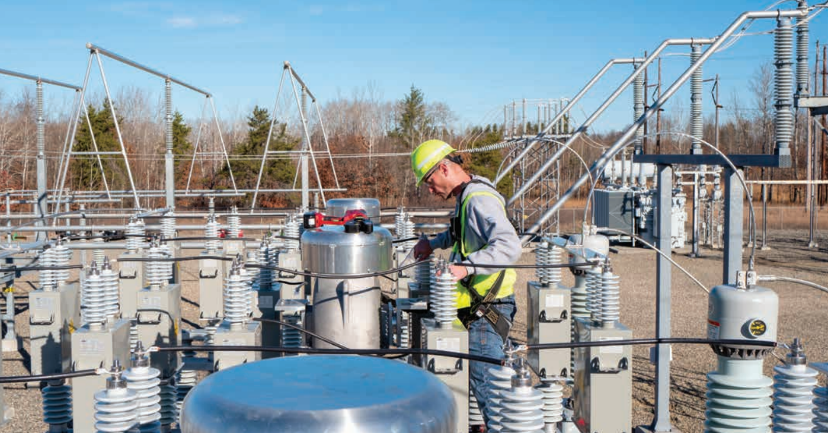
Surrounded by the northern Minnesota woods, Jason Bjerke, Minnkota senior technical maintenance technician, adjusts ripple injection equipment at the Wilton substation.
