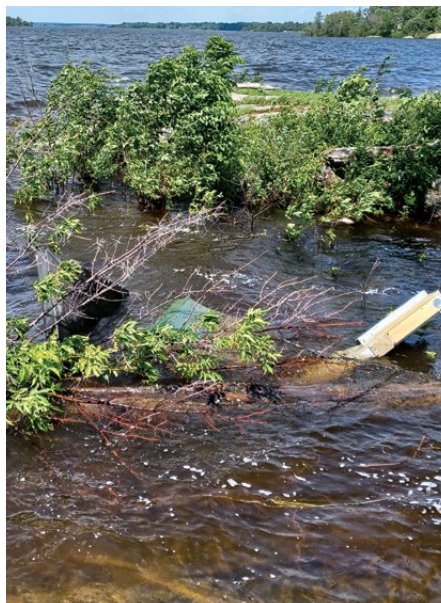
Transformer and meter pedestal waterlogged
