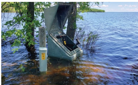
Primary voltage junction box submerged in water
