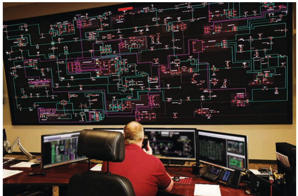
The distribution automation project will help provide power system operations personnel like Mike Bedney with more information from the substations across Minnkota’s system.
