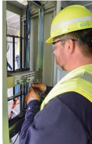
Jason Johnson, senior technician, completes telecommunications wiring work as part of the distribution automation project.
