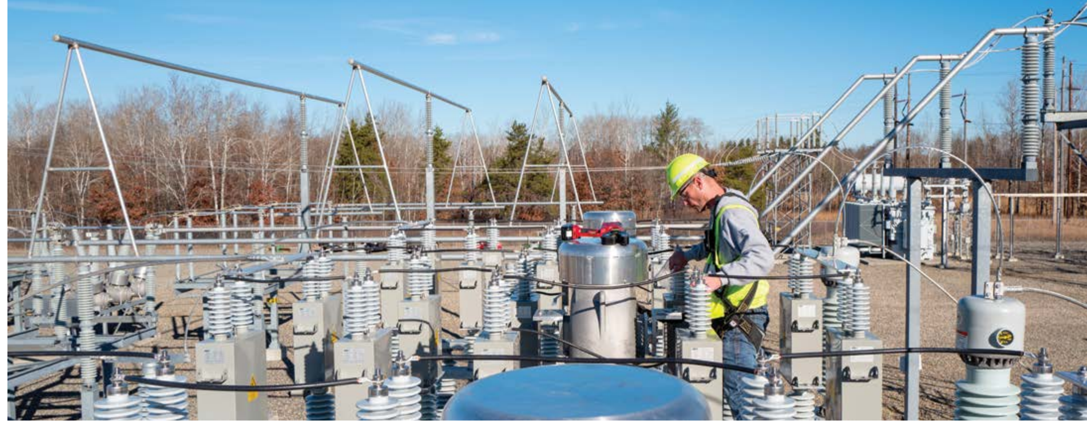
Surrounded by the northern Minnesota woods, Jason Bjerke, Minnkota senior technical maintenance technician, adjusts ripple injection equipment at the Wilton substation.
