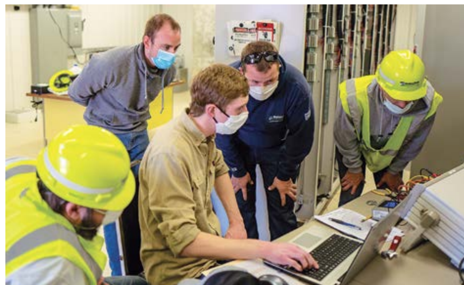
(Left to right) Joe Hensel, Patrick Rickenbacher, Nick Gellerman, Jared Thompson and Jason Bjerke work together to tune the new ripple injection system at the Wilton substation from the adjacent control house.
