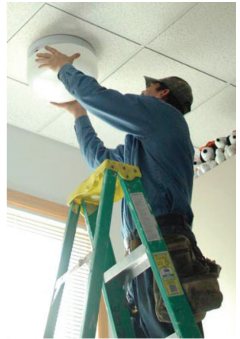
Red River Valley Co-op Power load management technician Paul Karsnia changes out light bulbs at the Hendrum Elementary School.
