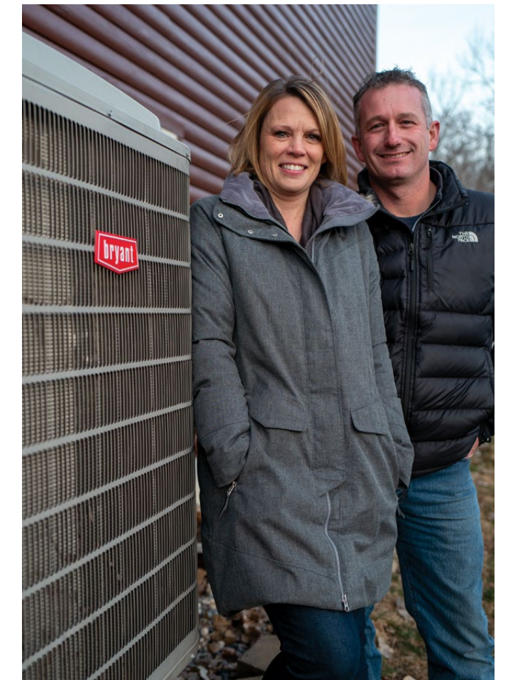
Co-op members Mike and MindyJo Halvorson received electrification rebates for the installation of their cold-climate heat pump.
