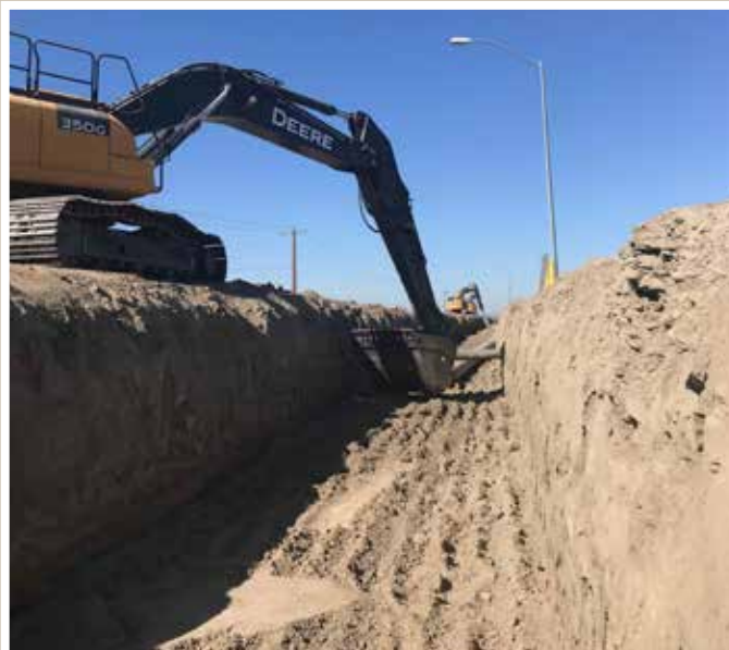
The lead machine is pulling and guiding. Two more pipes to go. Fun times!
