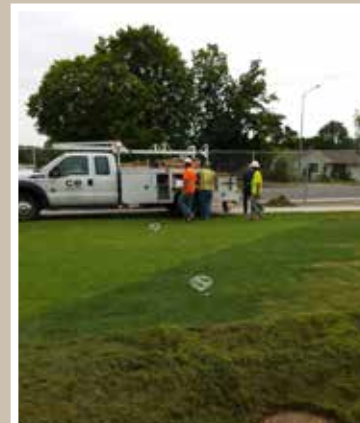
Finishing touches on some sod surrounding the green we cut through. You can still see where we replaced the green sod as well.
