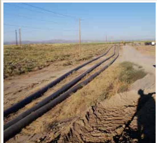
Three pipes ready to be installed in the ditch and one long shadow taking pictures!
