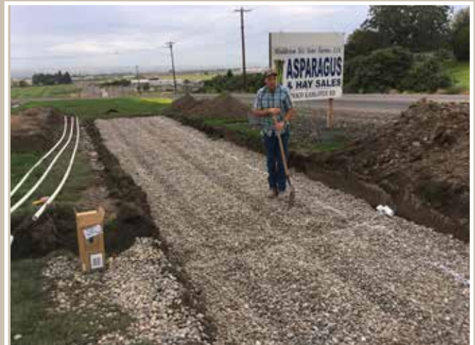
Greg pauses while prepping this leach bed for pipe installation. Congrats to Middleton's on their latest expansion. We can't wait to come check it out!
