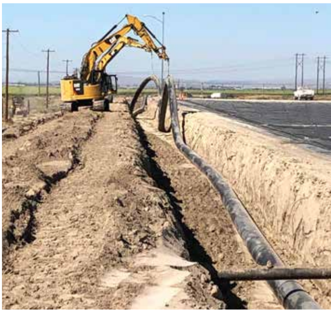
Phase 2 of installing 20" HDPE is a careful coordination of three excavators. Then into the ditch it goes.
