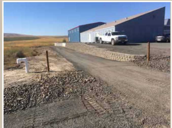
Our thanks to Harvest Heights Church for contracting with C&E to build their new multipurpose room (building in back). A special thanks to Circle K Enterprises, Brashear Electric, Total Energy Management and Dakota Concrete. We couldn't have done it without you!
