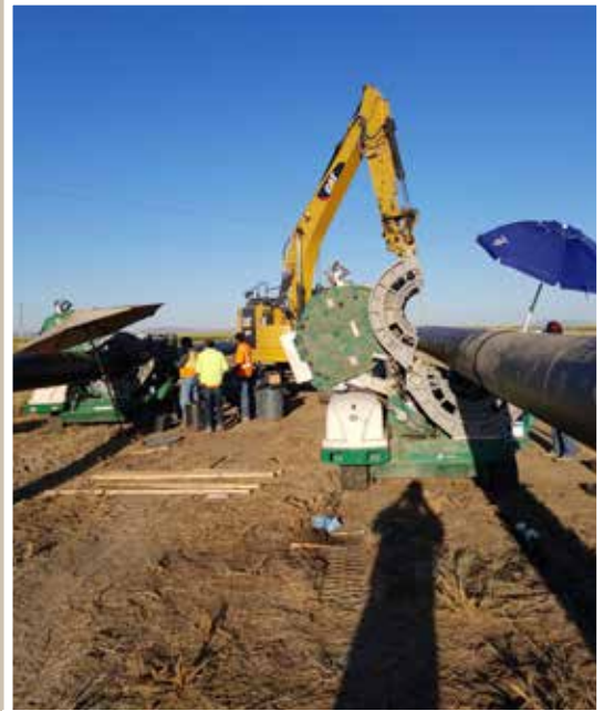
About 25,000 feet of 20" HDPE pipe to weld together in a short time frame means two fusion welding machines on site!
