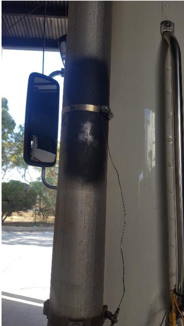
Figure 6: Exhaust pipe with heat shield remove. The hot component test surface has been prepared with matt finish ready for thermo camera/gun testing. In this case, a clamped thermo couple was also used to validate the testing approach. Note: in practice only one test method is required.
