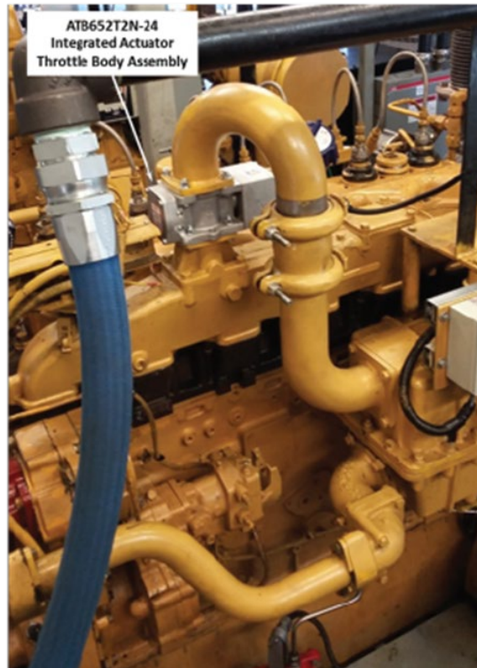
GAC ATB652T2N-24 Installed
