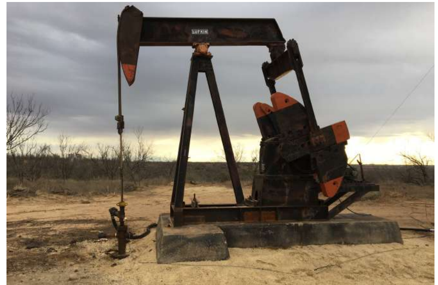
Typical pump jack on our wells.
