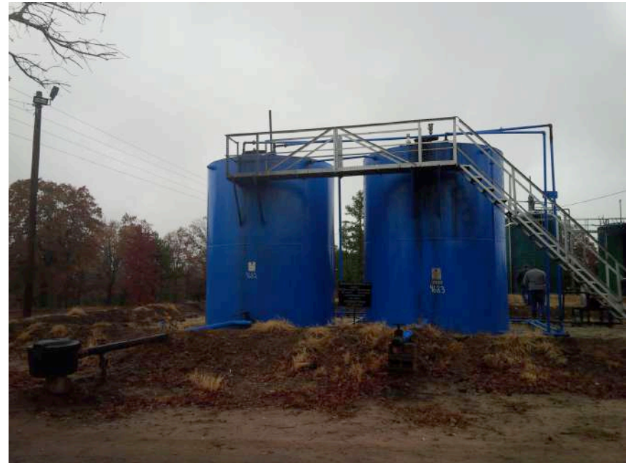
One of six tank batteries Nostra Terra owns.
