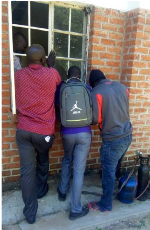
Here, we were making sure the class for the lab is well secured. Fine tuning the window panes.
