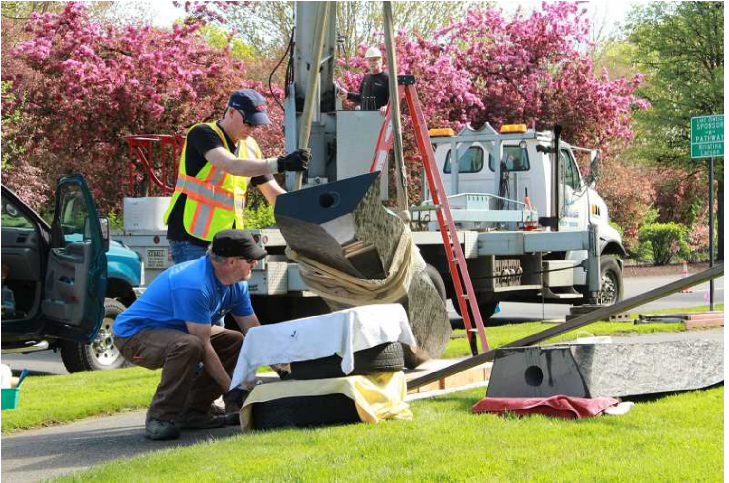
PMG PHOTO: SAM STITES - Haslett (front left) guides one of the 2,000-pound basalt columns onto cushions while installing it along Kruse Way in April.
