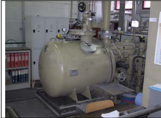
Figure 1- Industrial VIM plant
