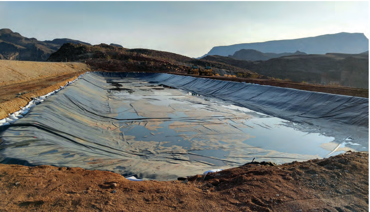
FIGURE 1 A 60-mil (1.5-mm) EIA/KEE geomembrane for a secondary containment application with a soil cover
