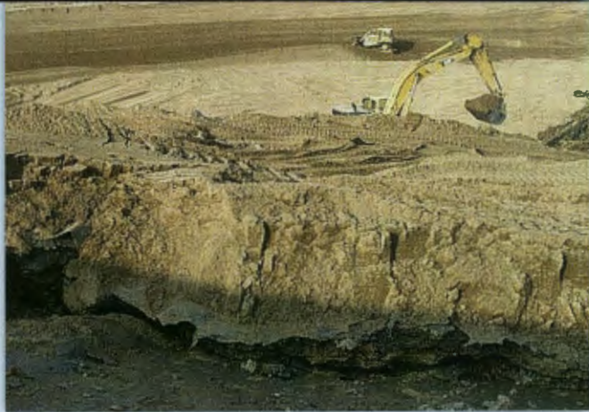
Figure 4. Slide surface and torn geomembrane.
