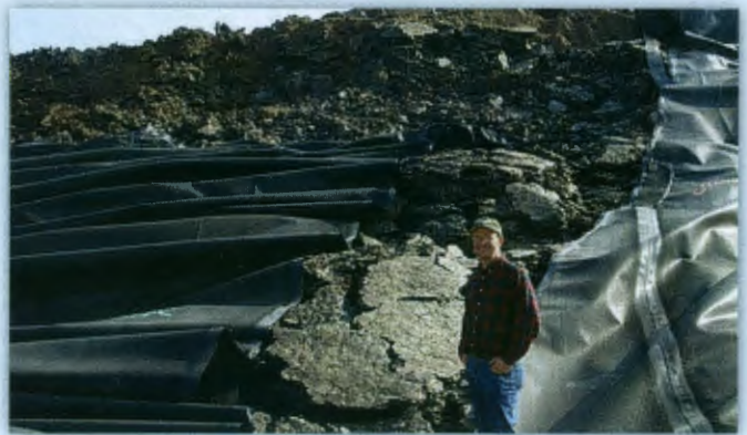
Figure 3. Failed slope and damaged geomembrane.
