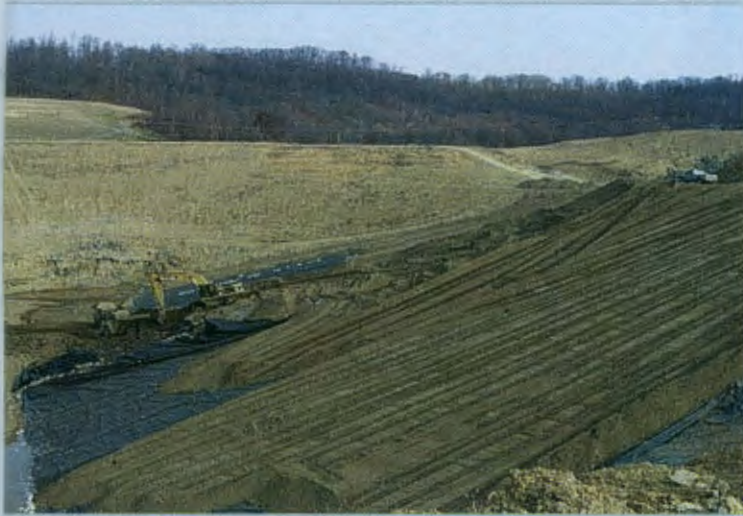
Figure 2. Overview of sideslope and protective sand placement on geomembrane from top of slope to bottom.
