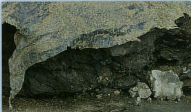
Figure 5. Close-up of torn geomembrane which shows slide surface is below geomembrane/CSL interface.
