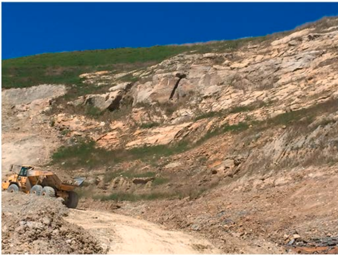
Fig. 11. Relatively smooth (non-benched) rock slope behind the RSS structure, after removal of slide debris. (Photo credit: Ryan R. Berg).
