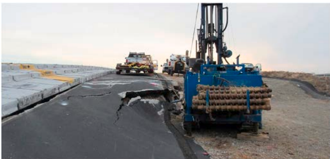
Fig. 5. Deformation at top of RSS structure and within the reinforced soil zone, approximately 1 month prior to collapse. (Photo credit: CWVRAA).
