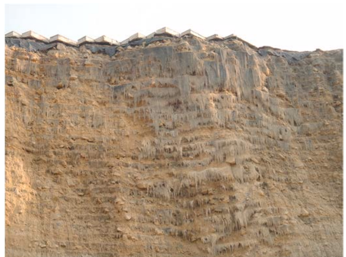
Fig. 7. Photo of 30 m high failure scarp through the reinforced mass. (Photo credit: Ryan R. Berg).
