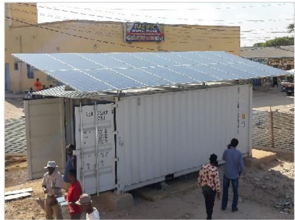
Cold room for fish, Off-grid in Hergeisa, Somalia - 2019
