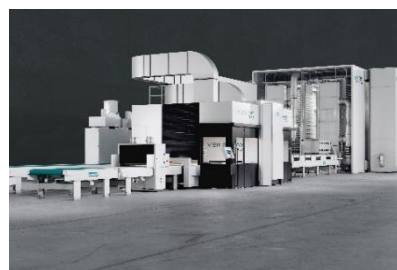
Insourcing painting line in Roggwil (CH)
